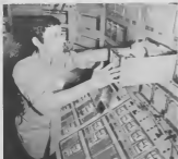
Assigned to Instrument Section, electrical student Mariano Arands observes intricate panel recorder box at the Refining Control Center.
